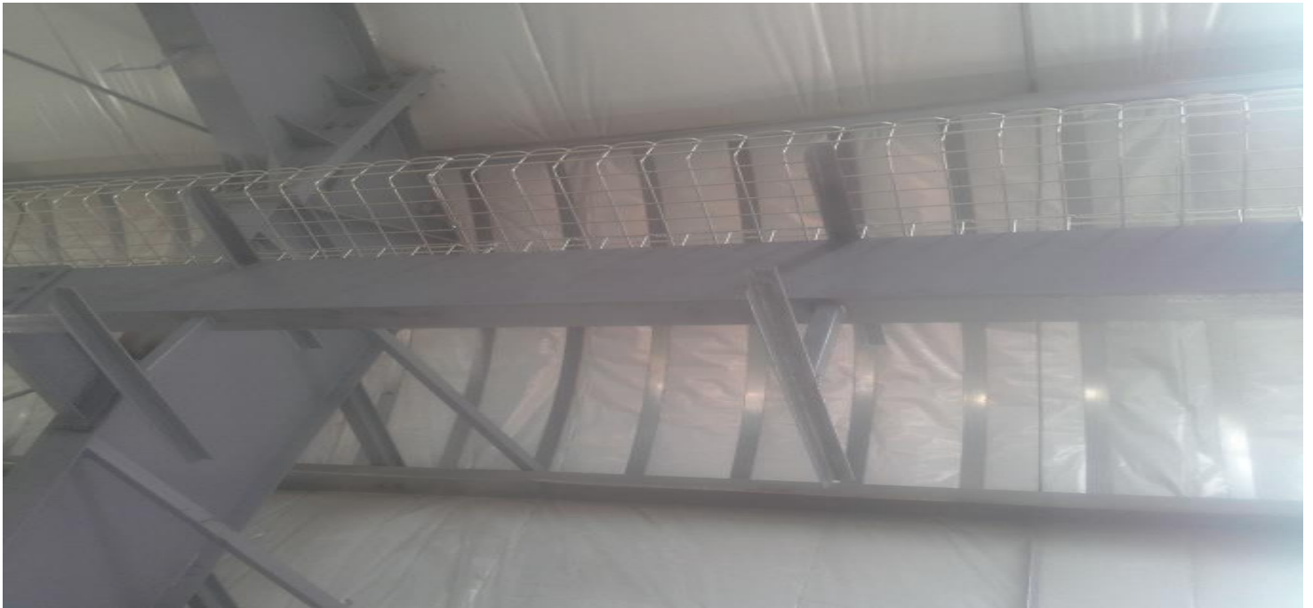
Cable Tray: for using underground cable so better using system in Cable tray system.
