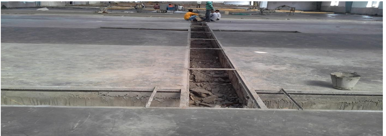
Under Ground Cable System. For Mangalam Fabricator in Text pin Plant.
